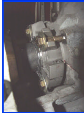
USS MONTEREY (CG-61) pump with split mechanical seal
